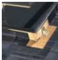
Installing roofing underlayment between the skylight frame and roofing material will help prevent condensation on the cladding and flashing.
